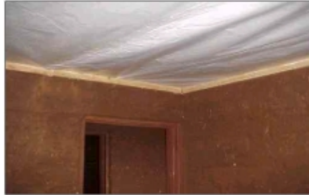
Figure 10 Innovative ceiling products can reduce the investment by 50%. Photo: (Pal, Geurtsen et al. 2000).
