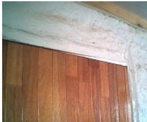
Figure 9 Air gaps between the door and doorpost lead to excessive heat losses
